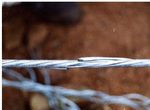
Figure 1. Photograph of ground wire (80sq. OPGW/AC) that was damaged by lightning.
