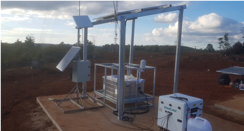
Figure 8: Example deployment adjacent to a met tower – Example deployment to perform WRA in Laos. The lidar is offset a few meters from outermost guy wire anchor. Beam CNR was closely checked during setup to confirm no guy wire interference. Photo courtesy of Impact Energy Asia Development Limited (IEAD).
