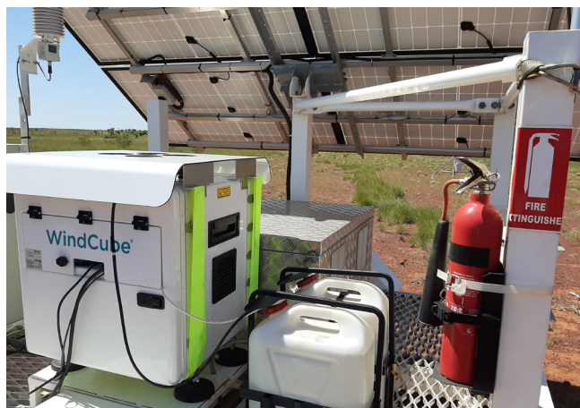
Figure 15: Sunshade atop of WindCube unit installed on a trailer in the desert – Sunshade and trailer installations reduce the exposure of the lidar to direct solar radiation.
